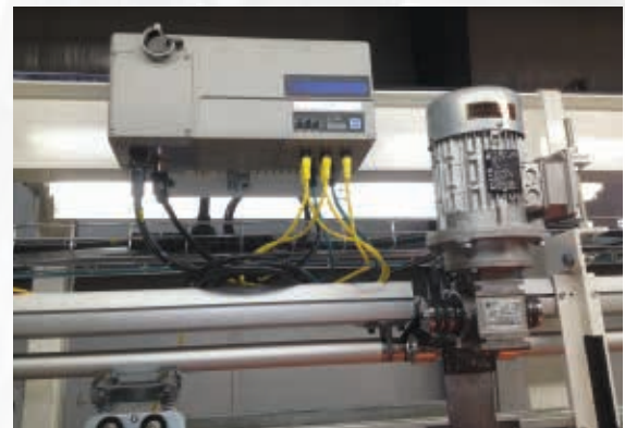
½ HP gear motor drive with motor controller.
